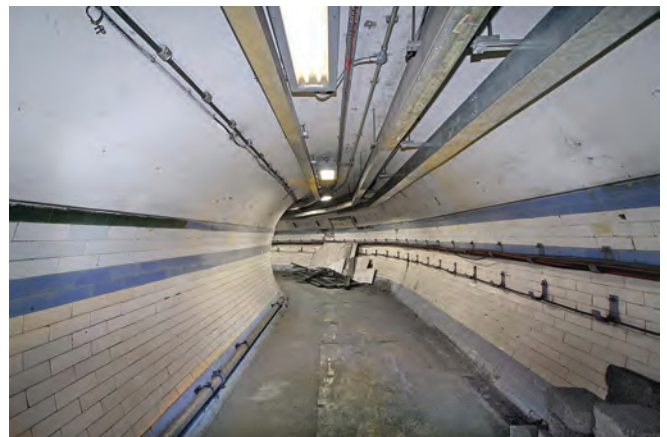
The 'out' subway at Dover Street looking towards the trains. The original subway tiles with the unique colour theme are still in good condition in much of the subway. In the distance on the right an original sign can be seen above the upper tile line indicating 'TO THE LIFTS'. Photo Nick Catford
